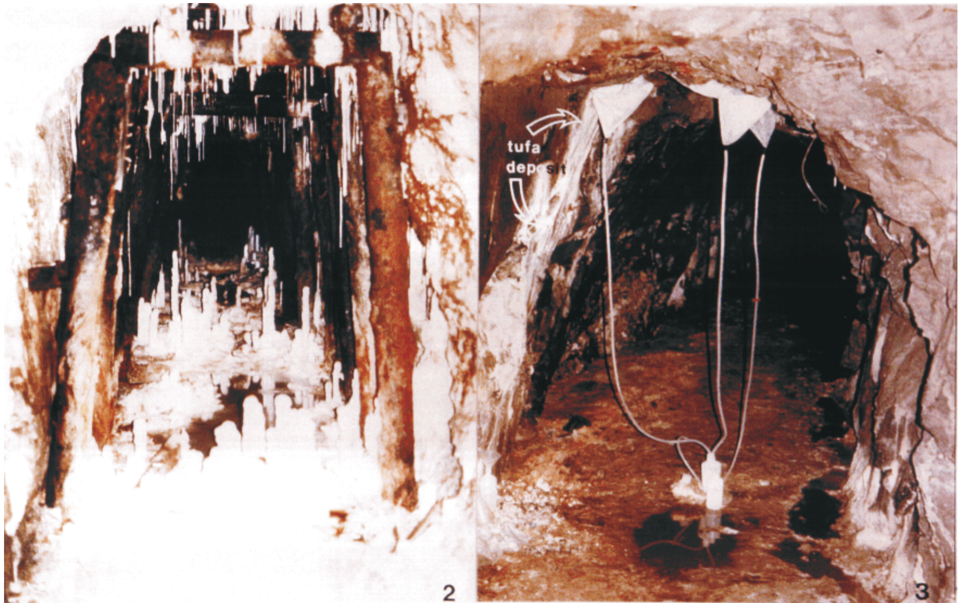
Plate 2 Principal zone of hyperalkaline groundwater seepage in Adit A6 showing extensive deposition of calcite-aragonite tufa/travertine on the adit walls. Sampling Site M1.
